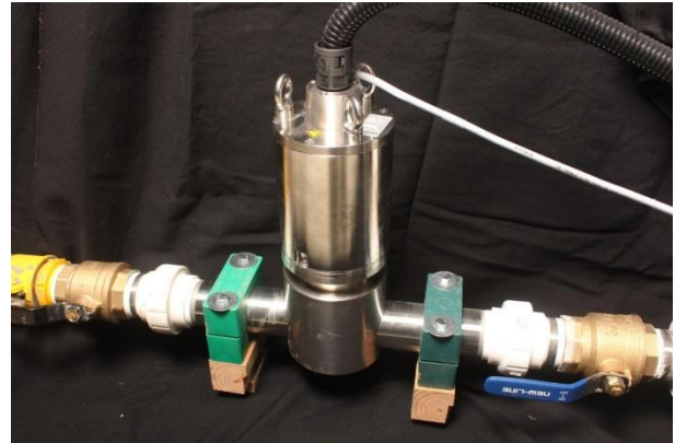
Figure 6. Custom pipe spool with NIR sensor head attached.
